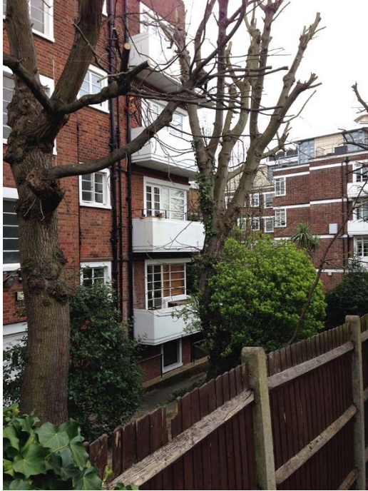
Photo A – View of Emmerson Court Elevation showing Corner to Draxmont elevation
